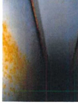
18) Rust bleedthrough on a roof plate.
