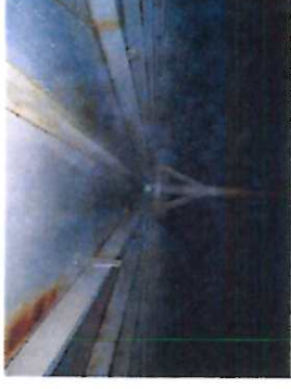
16) Wet interior roof with center column and channel supports. Rust bleedthrough present along stiffeners.
