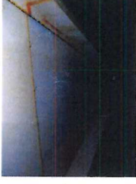
17) Rusting along the lap seams and roof plate to channel gap.
